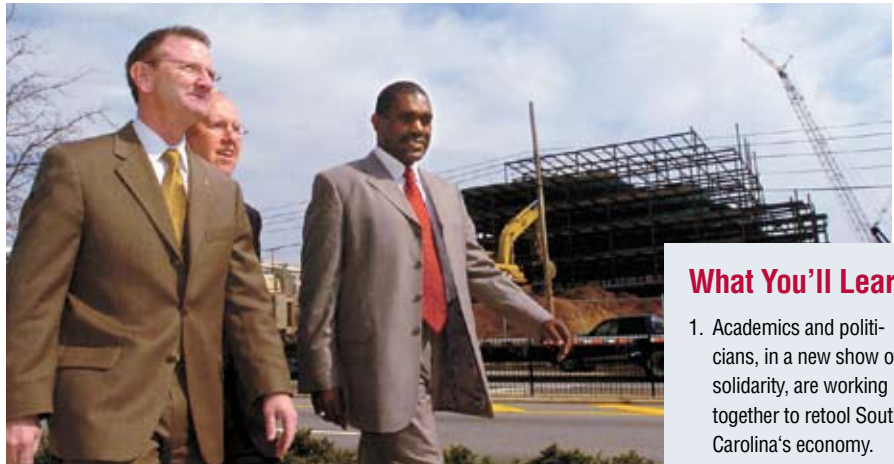
John Parks, left, executive director of USC's Innovista, Mayor Bob Coble, and Richland County Councilman Joe McEachern tour the Innovista construction site where Duck Creek Technologies will become the first-private sector tenant. Photo by Tim Dominick The State
